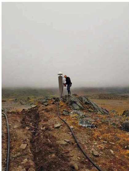
Figure 3: A researcher from the Warsaw University of Technology installing the antenna of the WUTH reference station
