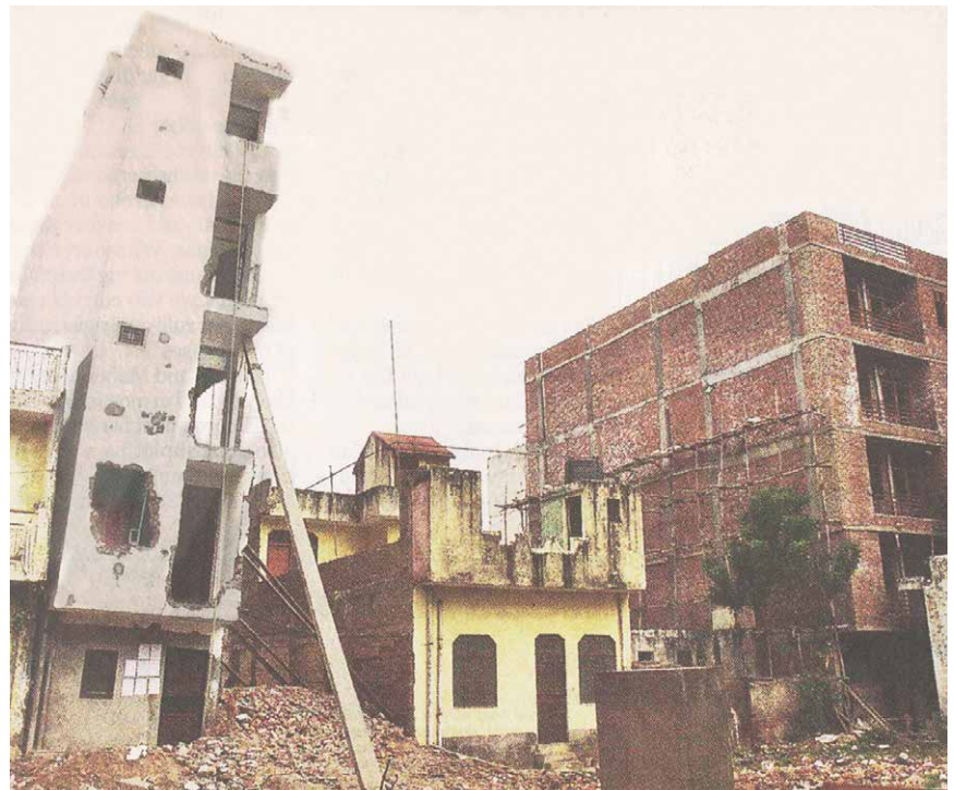
Fig 17: A leaning four-storeyed building at Mahavir Enclave in West Delhi
